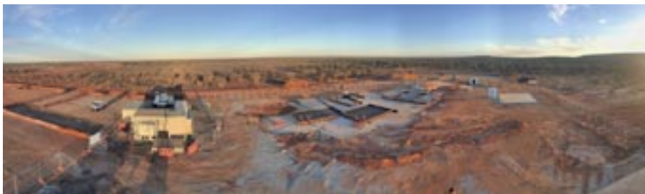
The foundations for the fans to be installed at St Barbara's Gwalia underground gold mine will consist of over 1,500 t of concrete and 300 t of steel
